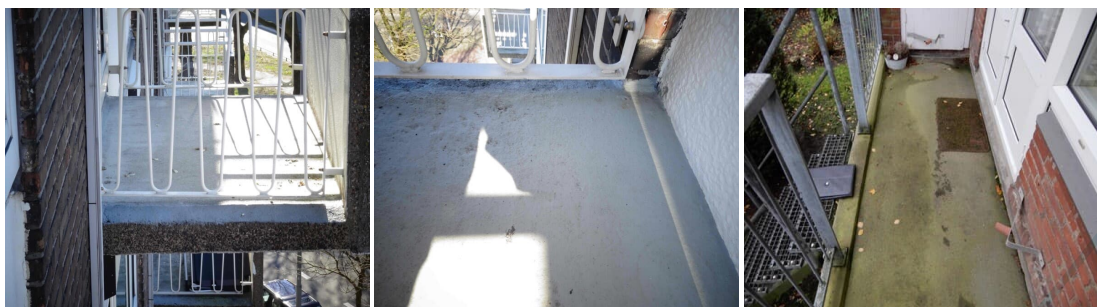
Foto 1: Coating intact, lichte vervuiling
